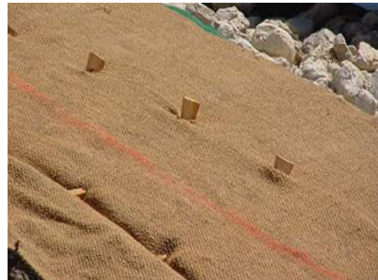
Fig. 6. Geotextile wool fabric mounted on the bank of a river as a support for the defence of the river [9]
