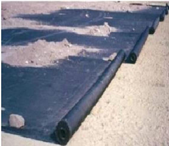
Fig. 4. Shore protection from non-woven geotextile mounted on the profiled slope of the river [10]
