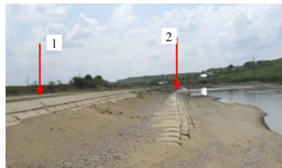
Fig. 14. General view of the left bank defence works: 1 - old concrete slab work; 2 - new work from geo-bags (photo, Sion, 2018)
