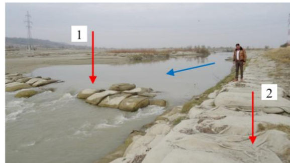
Fig. 13. Degradation of works from geo-bags on water action on the Moldova River: 1 - bottom threshold; 2 - shore defence (photo, Sion, 2019)
