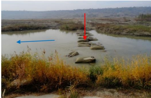
Fig. 11. Structural degradation of a bottom threshold made from geo-bags (photo, Sion, 2018)
